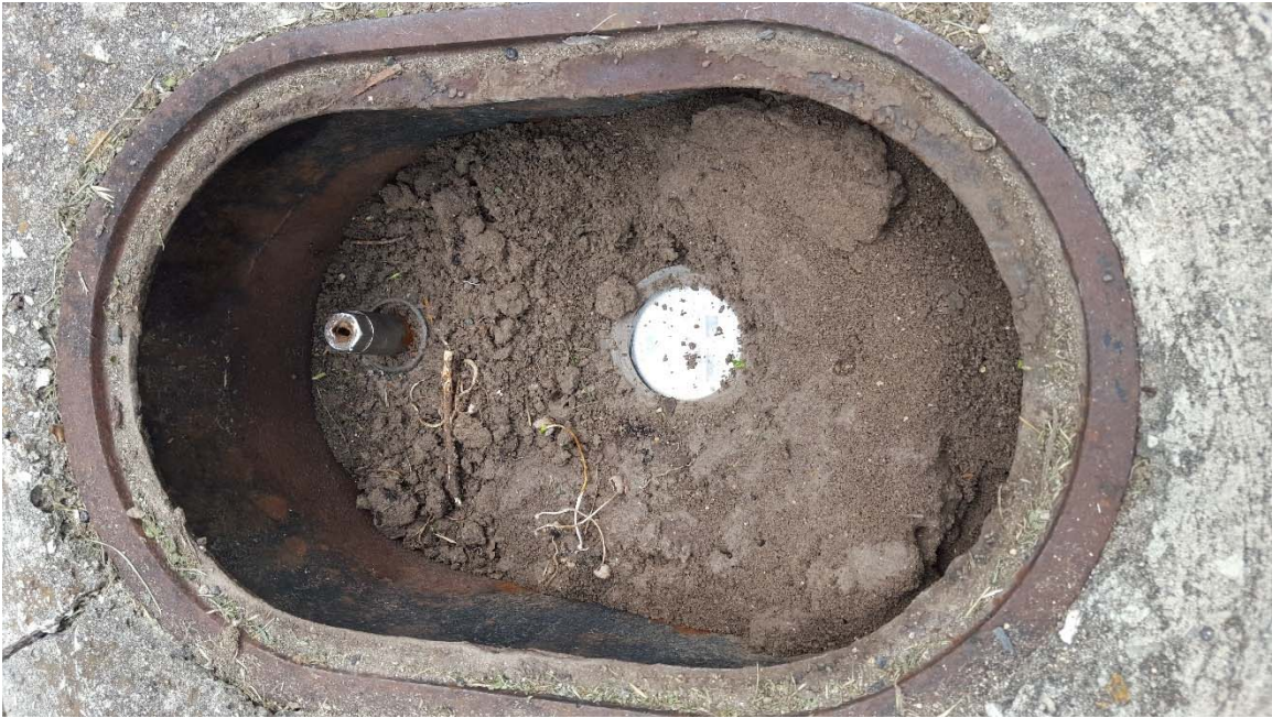
Photo 5 – Cycle 6 Meter at 8327 Robin Hill Dr (clean out excessive dirt / debris in meter box; verify curb stop valve is functional)
