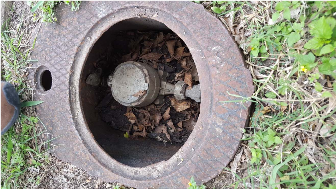
Photo 9 - Cycle 17 Meter at 211 Hoover Ave (replace meter box with SAWS standard to facilitate meter replacement and access to curb stop valve)
