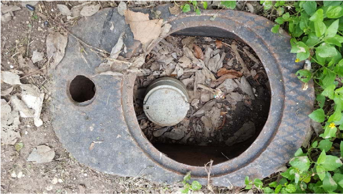
Photo 11 - Cycle 17 Meter at 330 Sims Ave (replace meter box due to poor condition and to facilitate access; clean out excessive dirt / debris in meter box)
