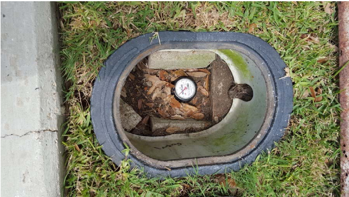
Photo 14 – Cycle 17 Meter at 1525 Keats St (clean out excessive dirt / debris in meter box; add meter yoke to raise meter closer to grade)
