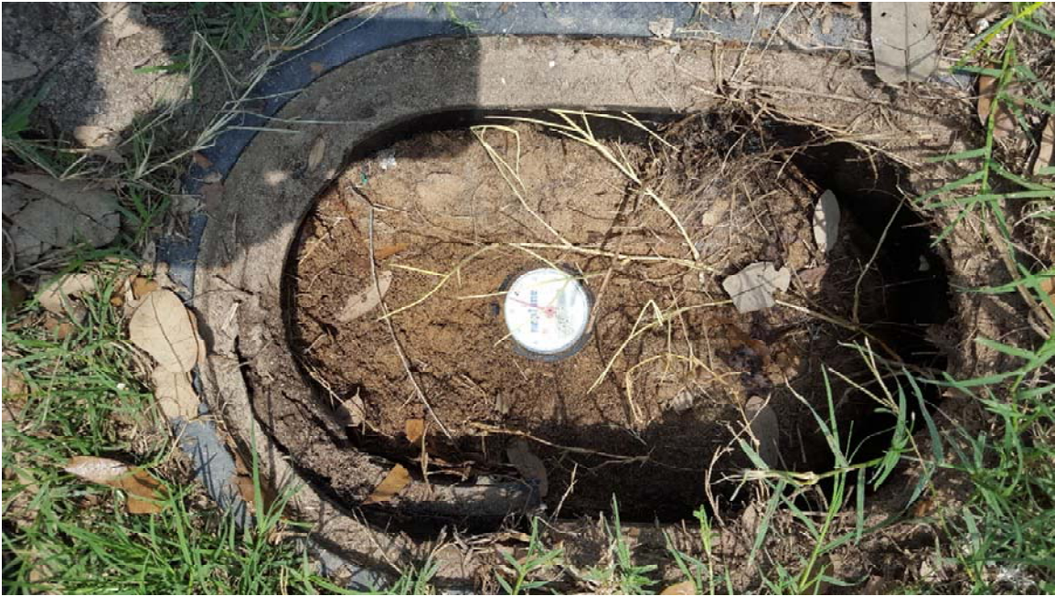
Photo 7 – Cycle 16 Meter at 168 Nueces Dr (excessive dirt / debris to be removed from meter box; replace meter box due to deteriorated condition)
