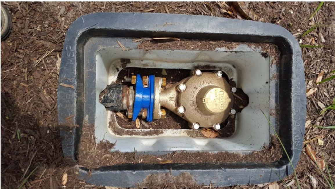
Photo 8 - Cycle 17 Meter at 134 Camino de Oro (tight fit for new 1.5-inch meter; meter box would be removed during meter replacement and should have been upsized)
