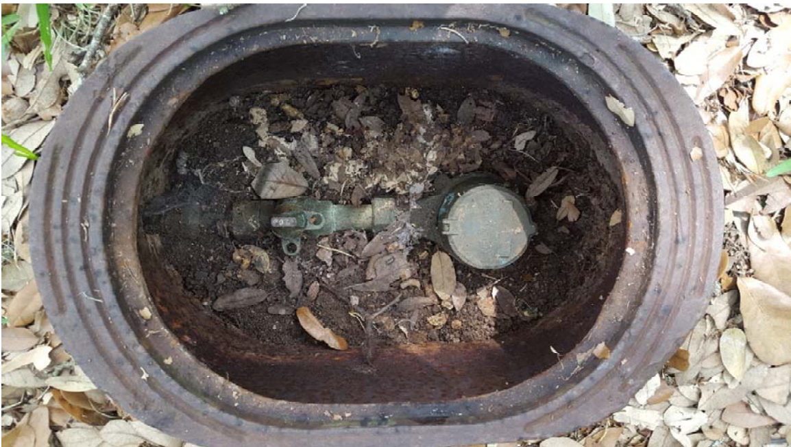
Photo 2 - Cycle 6 Meter at 106 Wisteria (may require meter box removal for new meter installation due to meter being offset in box)
