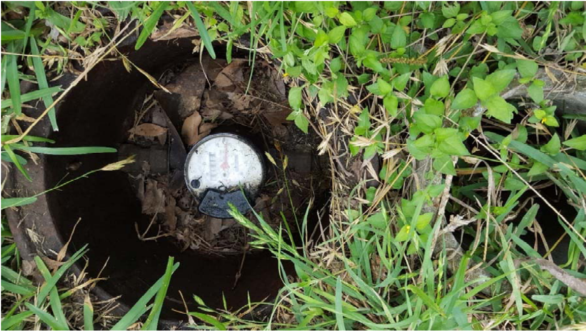
Photo 13 – Cycle 17 Meter at 478 E Hutchins Place (replace meter box with SAWS standard; clean out excessive dirt / debris in meter box)
