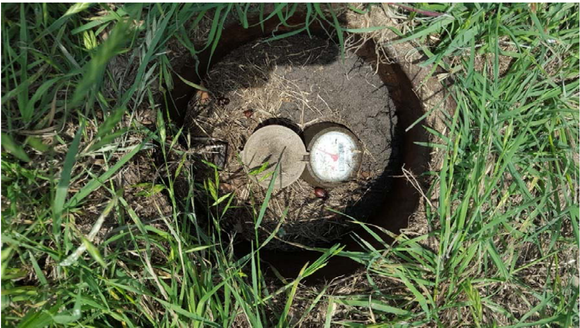
Photo 10 – Cycle 17 Meter at 315 Rosebud Ln (replace meter box with SAWS standard; clean out excessive dirt / debris in meter box)
