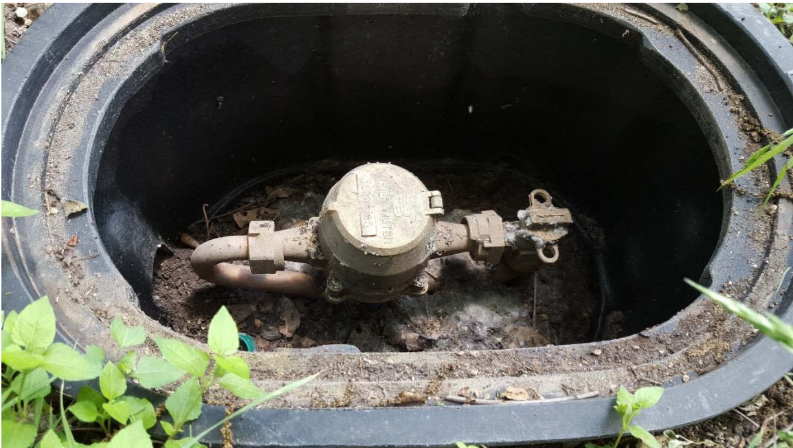
Photo 12 – Cycle 17 Meter at 1333 Stonewall Street (yoke required to raise meter closer to grade)
