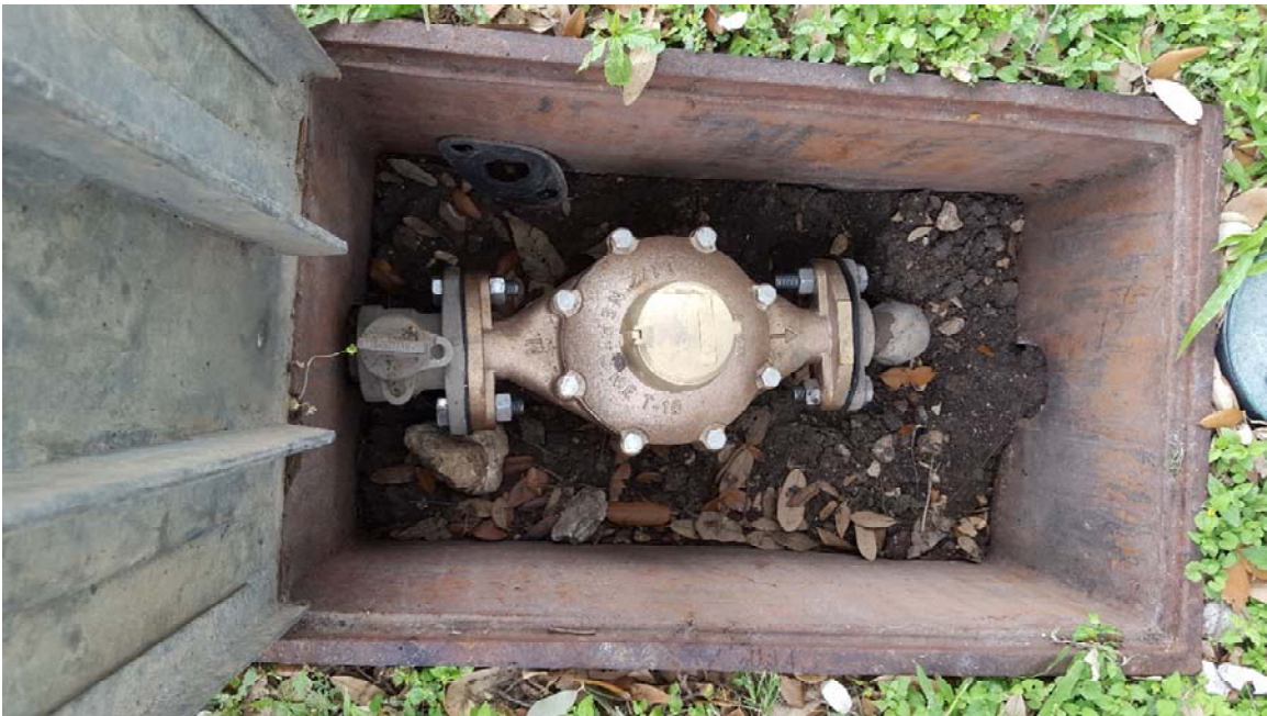
Photo 4 – Cycle 6 Meter at 4331 Vance Jackson (tight fit in existing meter vault for new 1.5-inch meter)
