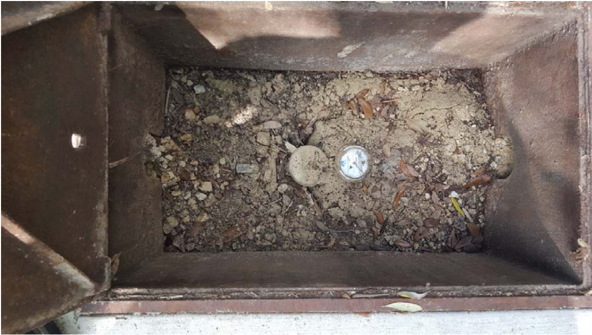
Photo 3 – Cycle 6 Meter at 2703 Marlborough Dr (clean out excessive dirt / debris in meter vault; add meter yoke to raise meter closer to grade)
